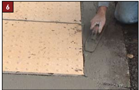
6 Finish surrounding concrete flush with panel. Install joints and finish to specifications.
