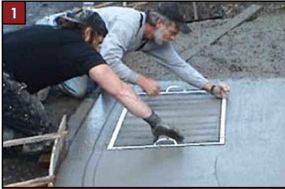
1 Pour concrete and finish to proper grade. Set INSTALaTACT® into fresh concrete 8" from curb line.
