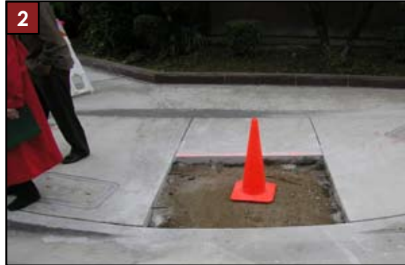
2 Prepare a well drained and properly compacted subgrade. Dowel into existing concrete as necessary. Oversize area minimum 2" in each direction.
