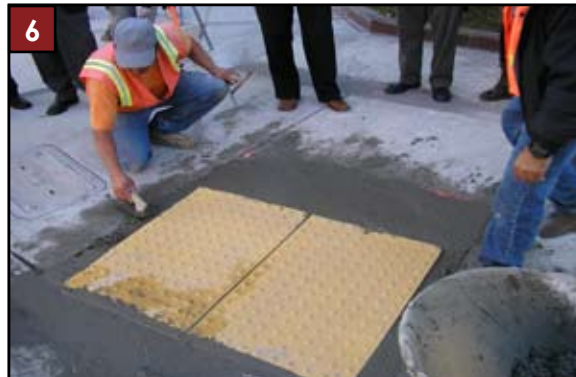
6 Fill perimeter with concrete, level with base of domes, edge panels, and finish to specifications.
