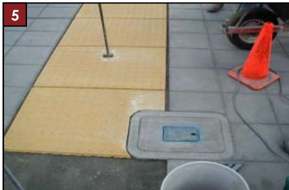
5 Install tactile panels with polymer modified medium bed thin set material. Wedge or flared edge of panel facing the curb.
