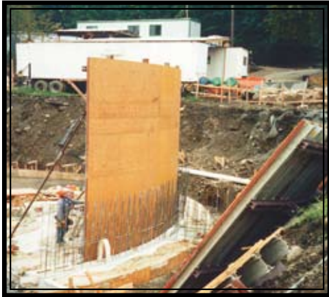
WWTP - WILSONVILLE, OR
